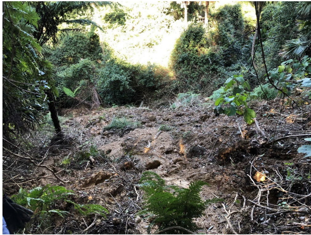
Terrain Unit 3 Photograph 5: Slip along steep section of Trail 22.
