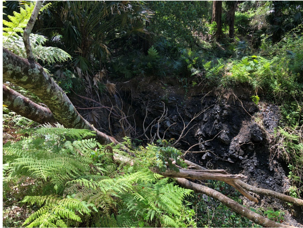
Terrain Unit 2 Photograph 21: Significant washout along the slip near a major drainage channel.
